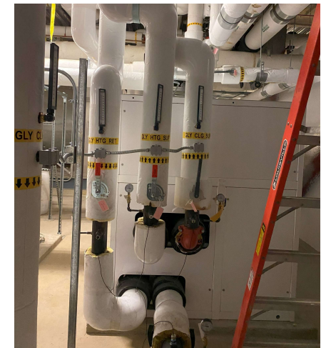
New supply and return piping
